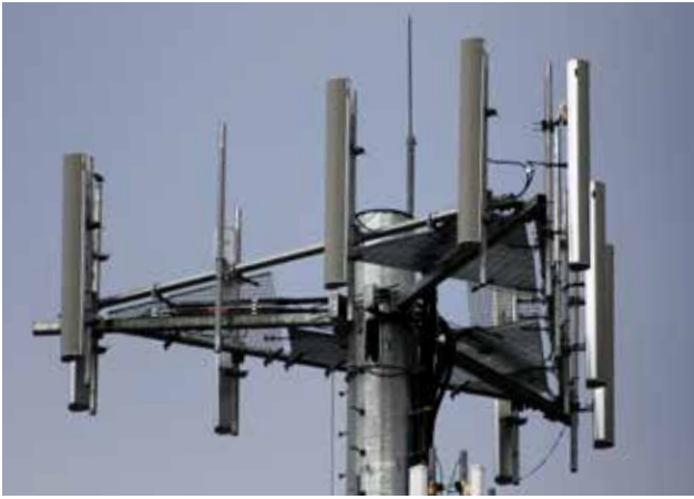
Figure 3.43: Mobile telecommunications mast
