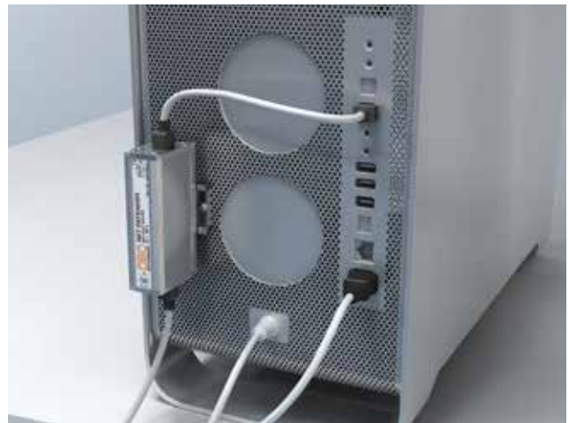
Figure 3.82: Suggested protection for terminal device. To keep the protection level low, the surge protection device uses the protective conductor of the PC case as the PE connection.
