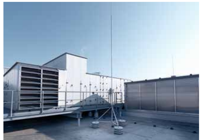
Figure 2.22: Insulated lightning protection with isFang
