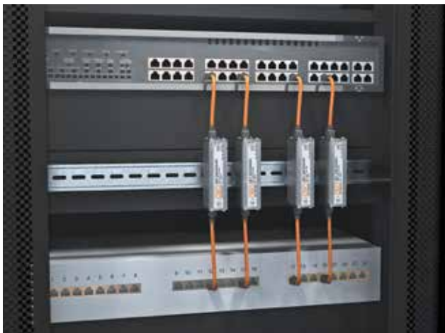
Figure 3.81: Suggested protection for switch with patch panel. The surge protection devices are earthed via the hat rail.
