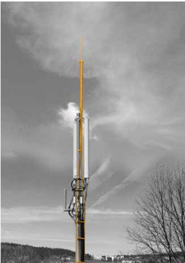
Figure 2.72: Cell tower with isCon® conductor
