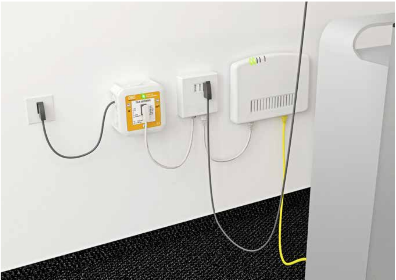
Figure 3.69: Protection of an ISDN + DSL connection with TeleDefender
