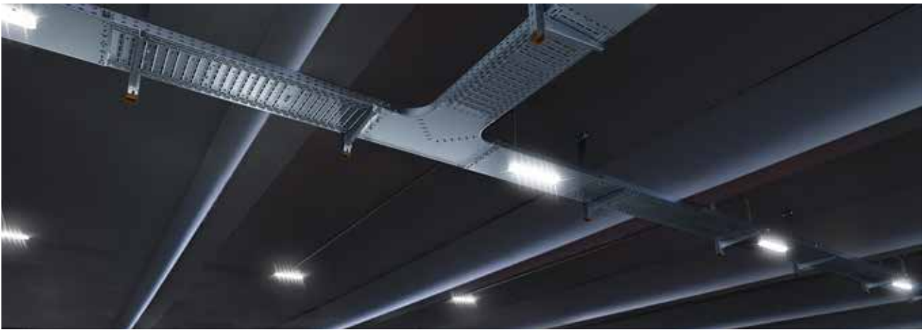
Figure 3.29: LED lighting system in an indoor car park
