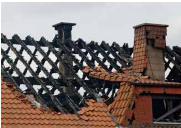
Figure 1.19: Building damage due to a direct lightning strike
