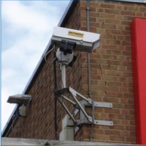
Figure 15. Violation of separation distance due to poor design and later additions to structure.
