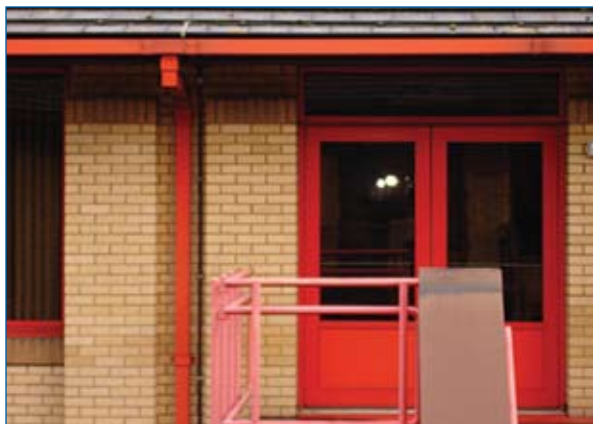
Figure 54. Example of poorly located down-conductor.
