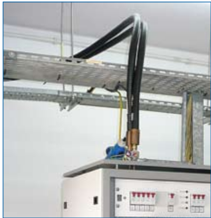
Figure 113. Incoming antenna circuits require protection.
