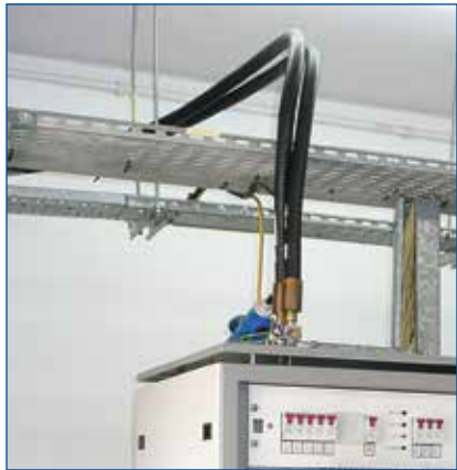
Figure 113. Incoming antenna circuits require protection.
