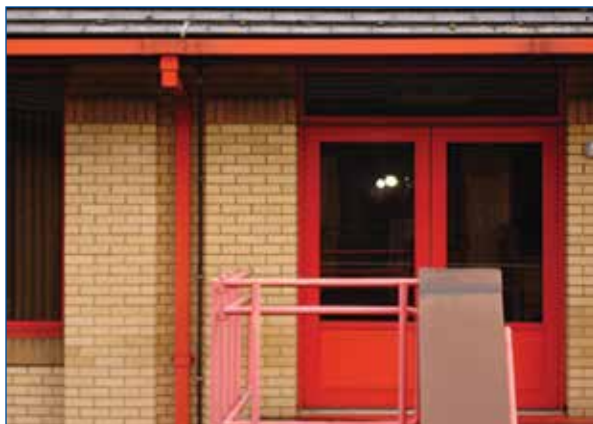
Figure 54. Example of poorly located down-conductor.
